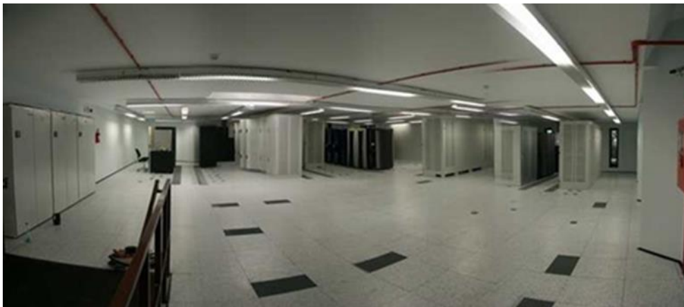
Figure 6: PSNC Server Room
